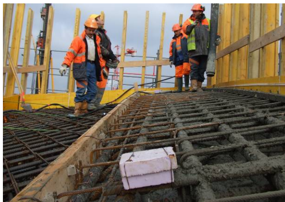
Figure 9: 1:1 mock up for transition zone between arches and slab areas during concreting
