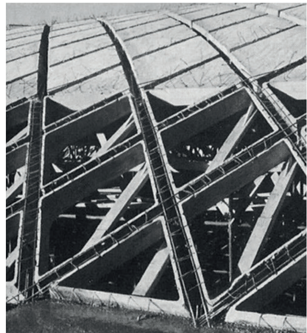
Figure 3 | Detail of the site during the construction phase of the ribbed pavilion vault. In the image it is possible to see the hollows for the casting of the ribs. Università di Firenze, Biblioteca di Scienze Tecnologiche (BST) - Archivi di Architettura, Fondo Pier Luigi Nervi (024-2783).
