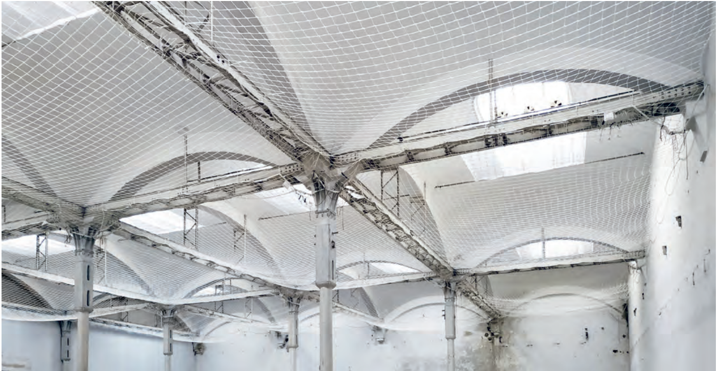
Interior de Can Bagaria (Fuente: Martín E., 2019) / Can Bagaria interior (Source: Martín E., 2019)
