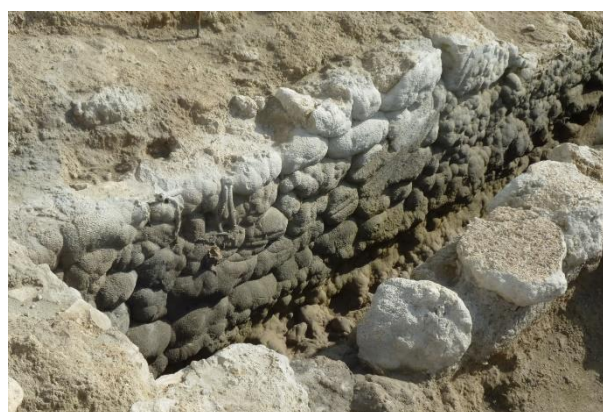
Figure 5: Photograph showing the mark left by the waterwheel on the stone wall.
